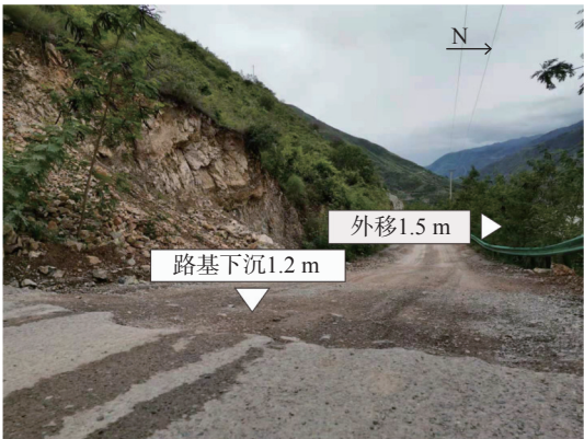
图 9 公路变形破坏 Fig. 9 Road deformation and failure
