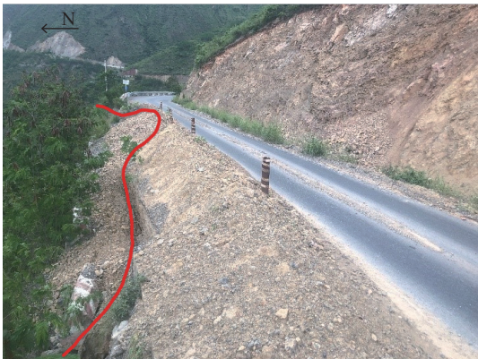
图 8 河口滑坡后缘变形 Fig. 8 Trailing edge deformation of Hekou landslide
