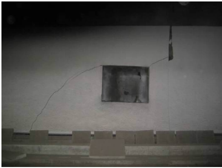
图 5 衬砌裂缝裂纹清晰 Fig.5 Clear trend lining crack
