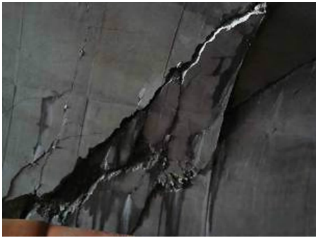
图 6 衬砌裂缝成网状交错 Fig.6 Crisscross networked lining crack
