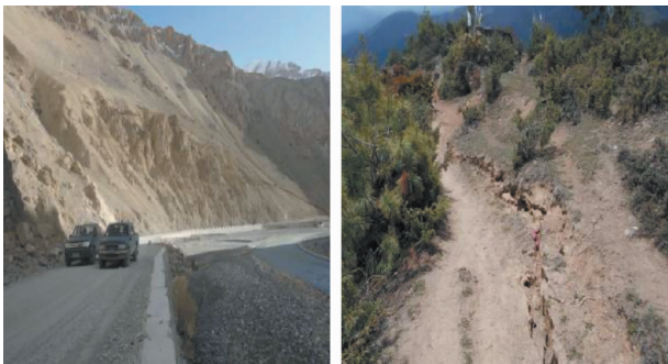
图 3 G216 沿线滑坡 Fig.3 Landslides along G216
